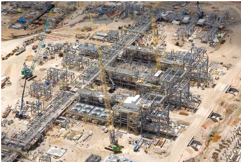
Hides Gas Conditioning Plant, March 2013
